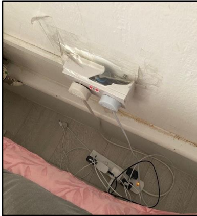
Broken electrical sockets with exposed wiring
