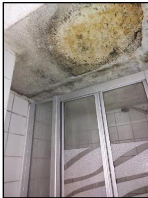
Damp conditions affecting shower ceiling
