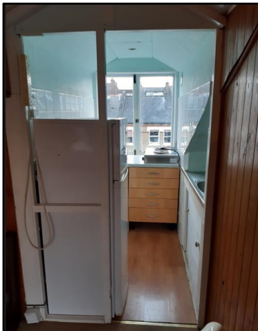
Fire safety issue from lack of door and partition to separate the kitchen from means of escape
