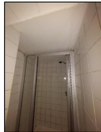
Cause investigated and replastered
