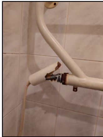
Exposed electrical component presenting risk of electrocution
