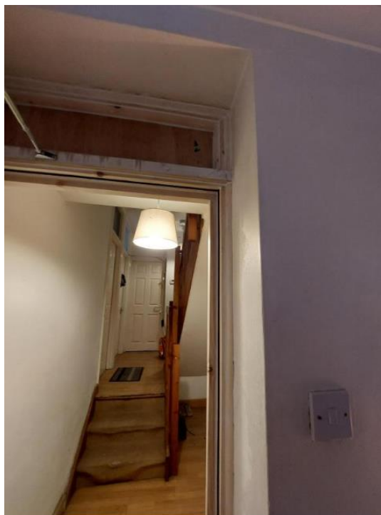
Inspectors found multiple breaches including faulty fire doors in homes managed by London Living Group (Image: Camden Council)
