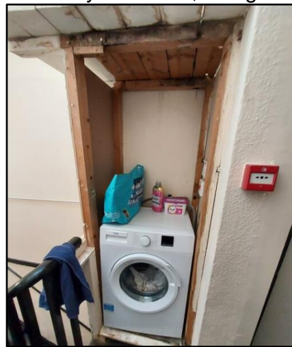
Washing machine in means of escape
