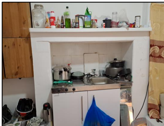
"Kitchenette" with inadequate space, worktop provision, food storage, power sockets and general layout.
